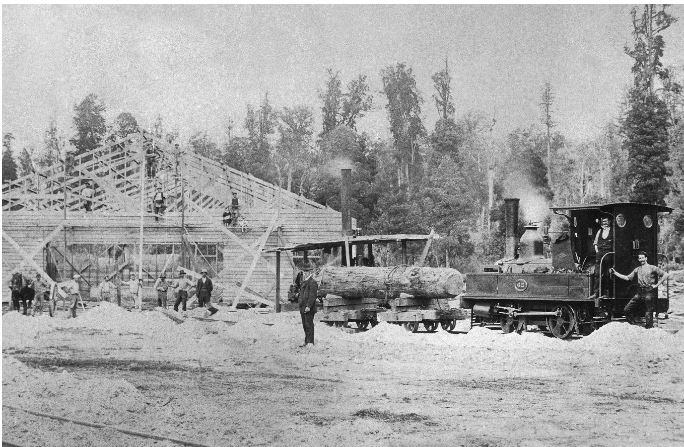
State Mill No 2 under construction late in 1910 at Bulltown. The mill manager, Gavin Weir, is standing centre foreground with the only other people known being James Galbraith who is standing in the cab of the “A” class bush lokey and Sid Henry standing on the cowcatcher.
