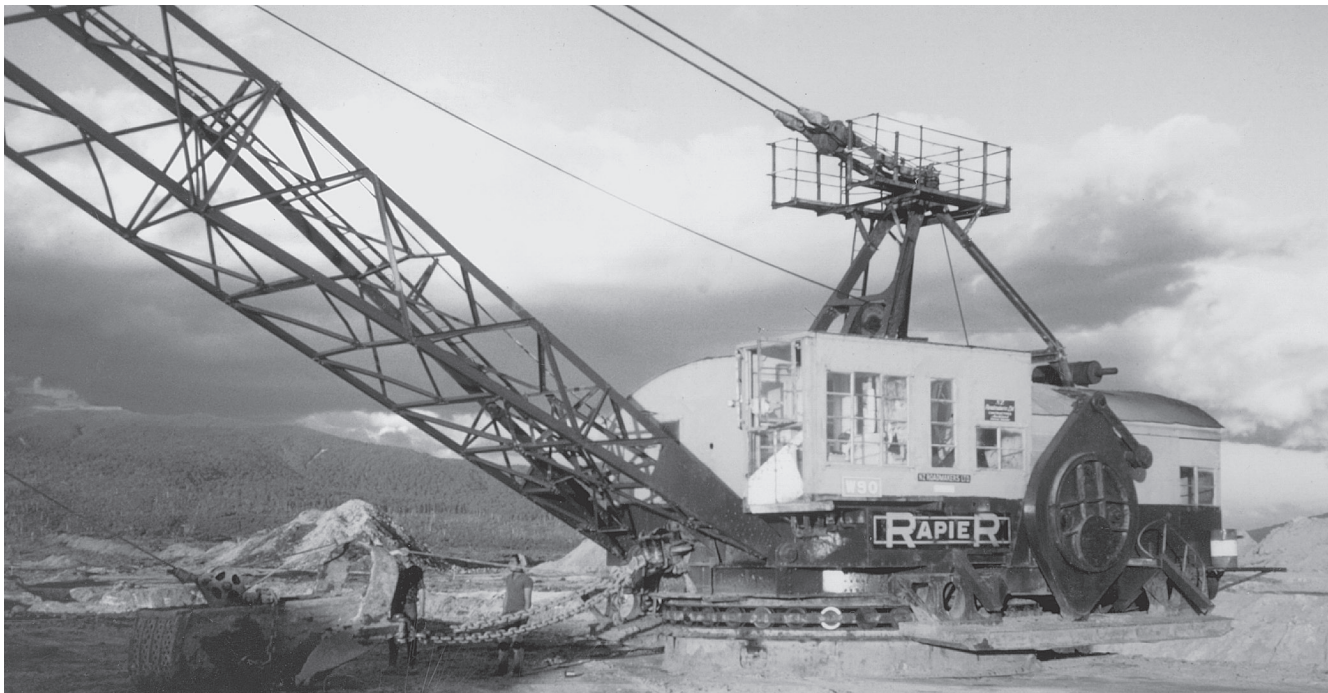
The huge Ransomes Rapier walking dragline which was used to dig some of the canals on the Western diversions. At the completion of the job it sat for several years on site before being dismantled and taken away.
